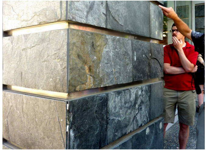
Figure 20.2.3 Slate used as a facing material on a concrete building column in Vancouver.
